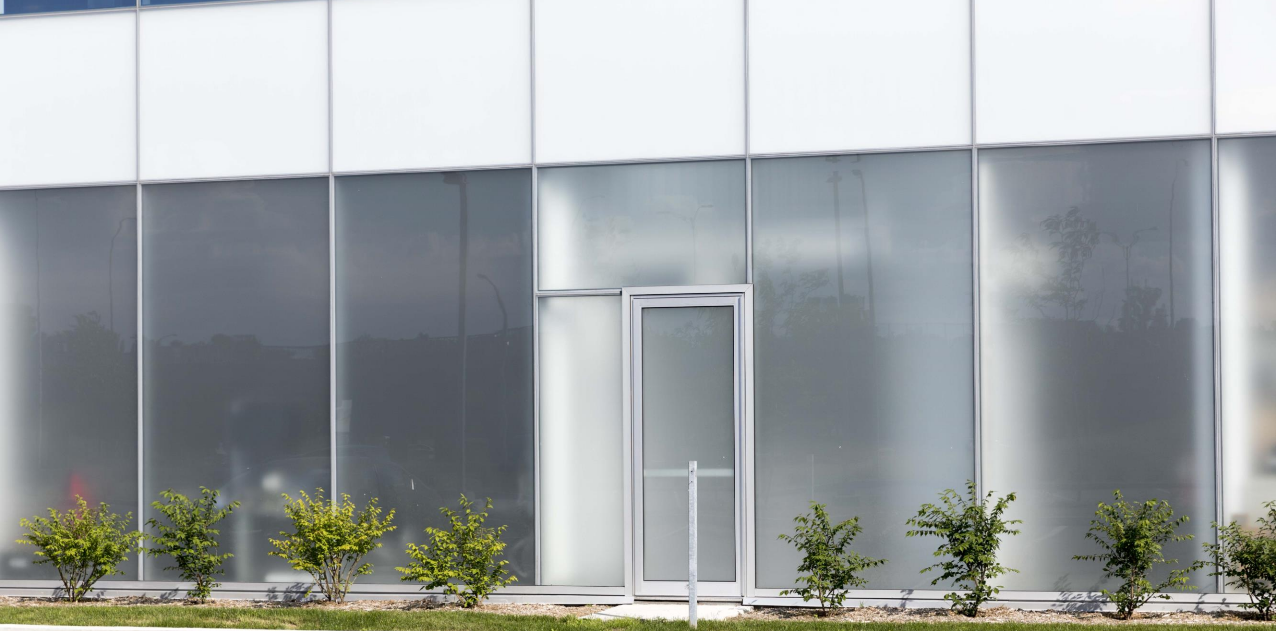
ABB Canada Campus (LEED® Gold Certified) – Montreal, QC 6mm Starphire Ultra-Clear™ glass Opaque finish on surface 2
