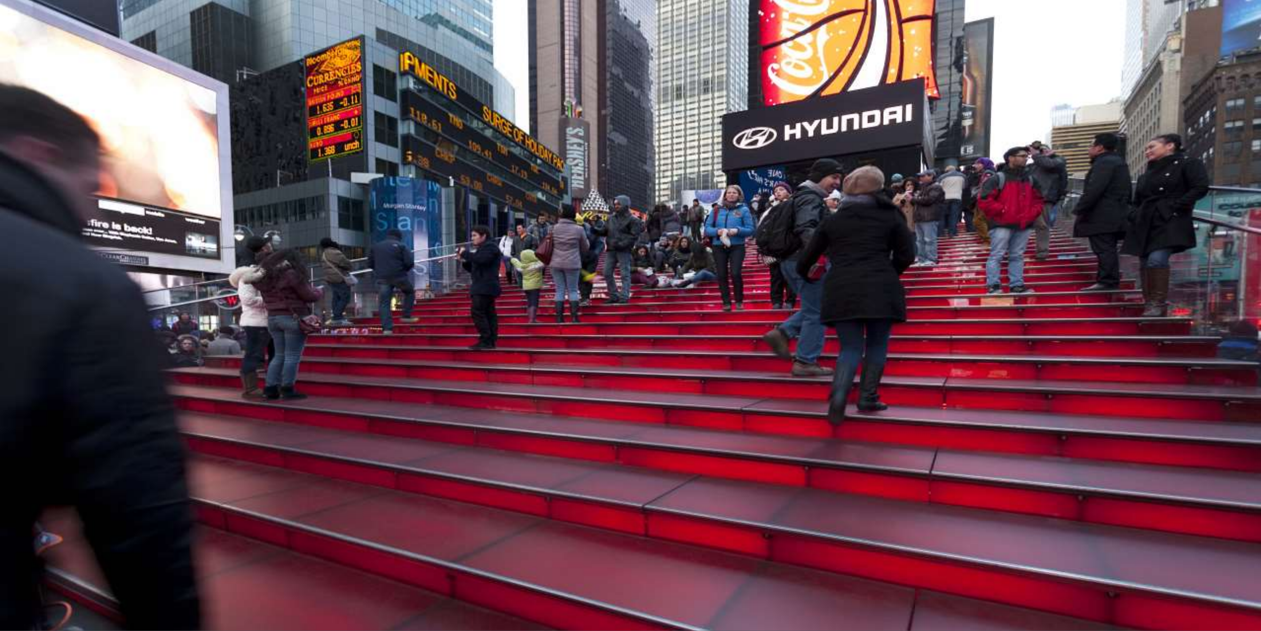
TKTS Stairs – New York (Times Square), NY 12mm Starphire Ultra-Clear™ Glass with Anti-slip Pattern, Tempered & Laminated
