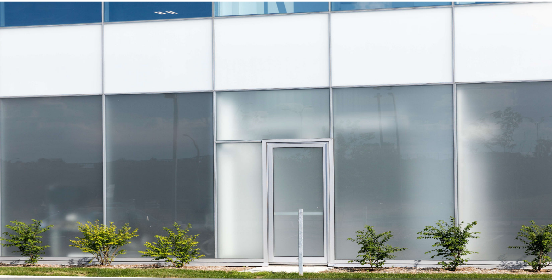
ABB Canada Campus – Montreal, QC IGU – 6mm low-iron acid-etched glass on surface 2, low-e on surface 3
